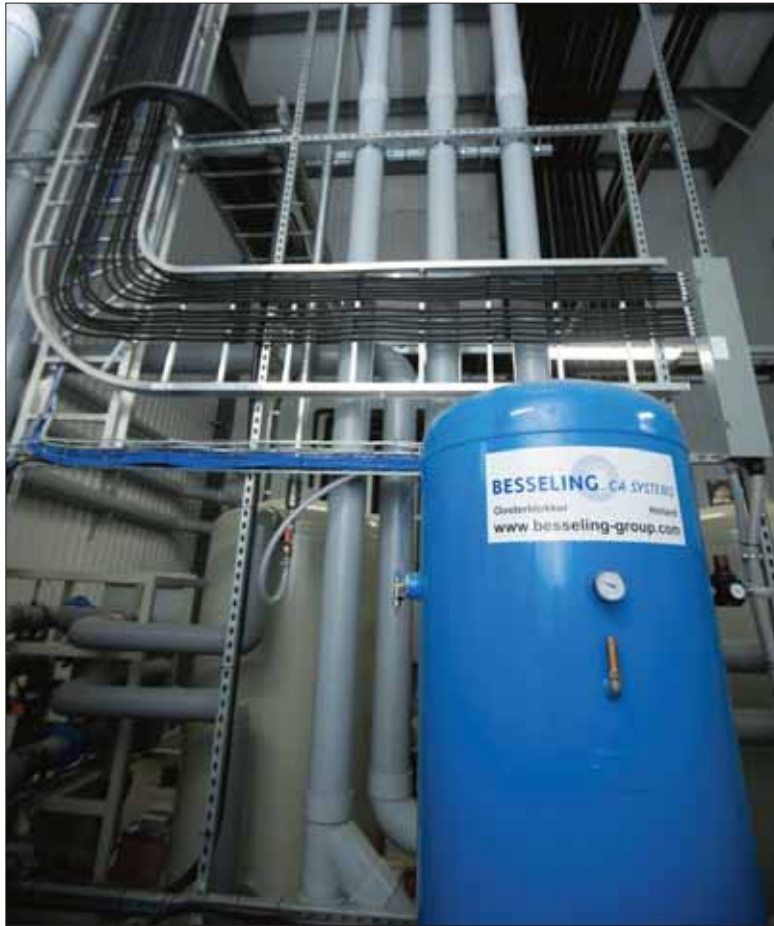
The Dutch expertise of Besseling CA Systems was contracted for the installation of controlled atmosphere rooms, panels and doors.
