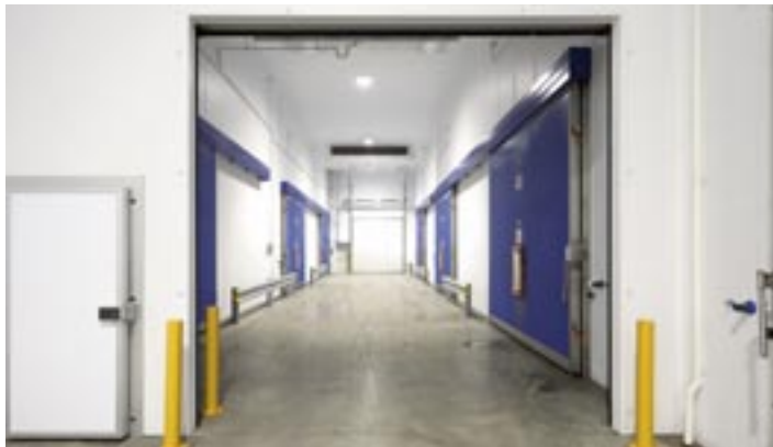
An internal view of the new fruit stores designed and constructed by Wealden AM.
